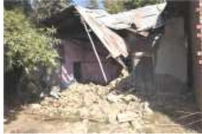
Damage caused by the disaster at Toubungkhok
