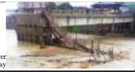
Temporary Chakpi River bridge swept away
