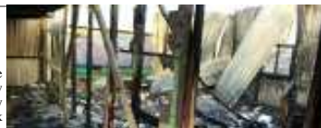
Burnt portion of the Administrative Block of New Public Higher Secondary School Khangabok
